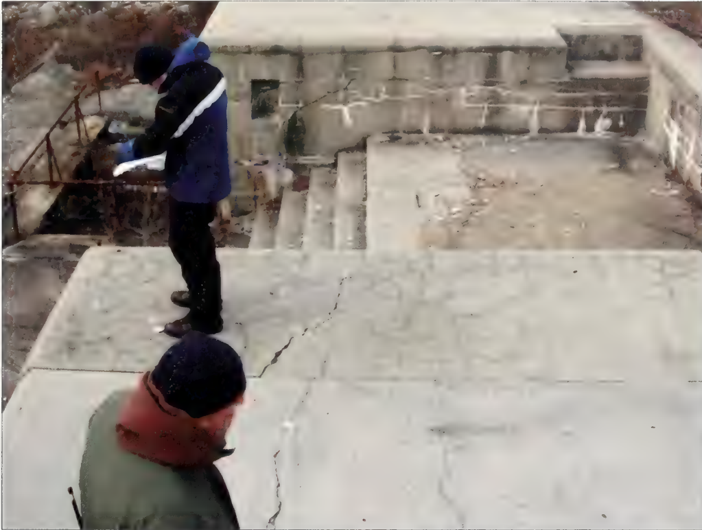
Figure 3.1. View looking west at gun platform #5, Battery Urmston. The gun platforms for emplacements #1, #2, #5, and #6 are T-shaped with full-width steps that lead up the long leg of the "T." At the north end of the platforms, narrow notches served as a recessed space to rest pillar mounted guns when not in use (Olmsted Center, January 2009).
